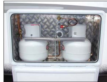
Dual 4kg gas cylinders stored in a side locker.
